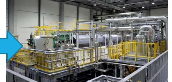
Single Alkaline water electrolyser stack, 10 MW
