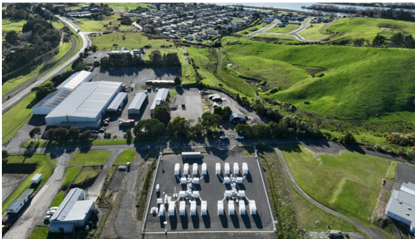
Rotohiko BESS (35 MWh, December, 2023) [ https://infratec.co.nz ]
